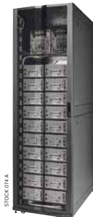
LI-ION BATTERY UPS with 20 hot-swap plug-in battery modules (model with 2 independent strings).
